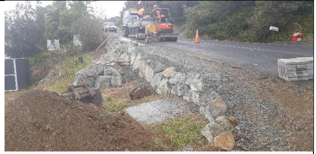
Cable Bay Block Rd rock wall to create width for the new footpath.
