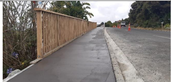
Cable Bay Block Rd 2 nd retaining wall with handrail and fresh pour before washing for exposed aggregate.
