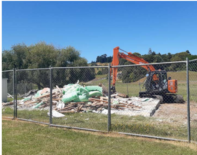
Contractors clearing out the remainder of debris following the demolition of three units at the Oxford Street, Kaitaia Village.
