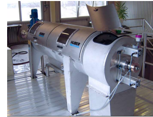
Solids dewatering mechanical
