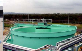
8 m diameter secondary clarifier
