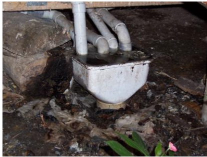
Backup to gully trap from clogged tank
