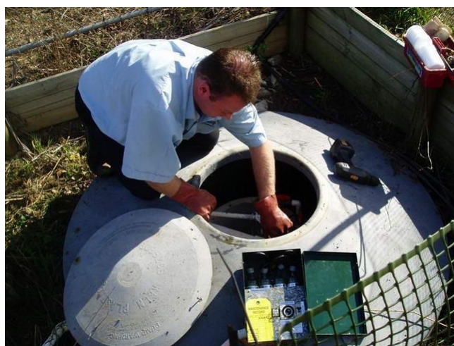
Servicing an advanced wastewater treatment unit
