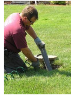
Lifting and hosing down effluent outlet filter
