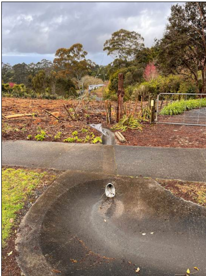
Figure 12 – Lot 2 water table outlet discharging onto site in uncontrolled manner at southern end
