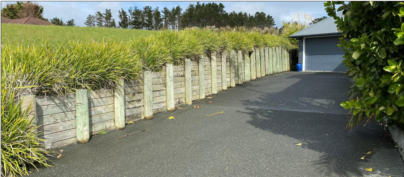
Figure 4: Site Photo – Overlooking the Neighbouring Retaining Wall to The West of Site.
