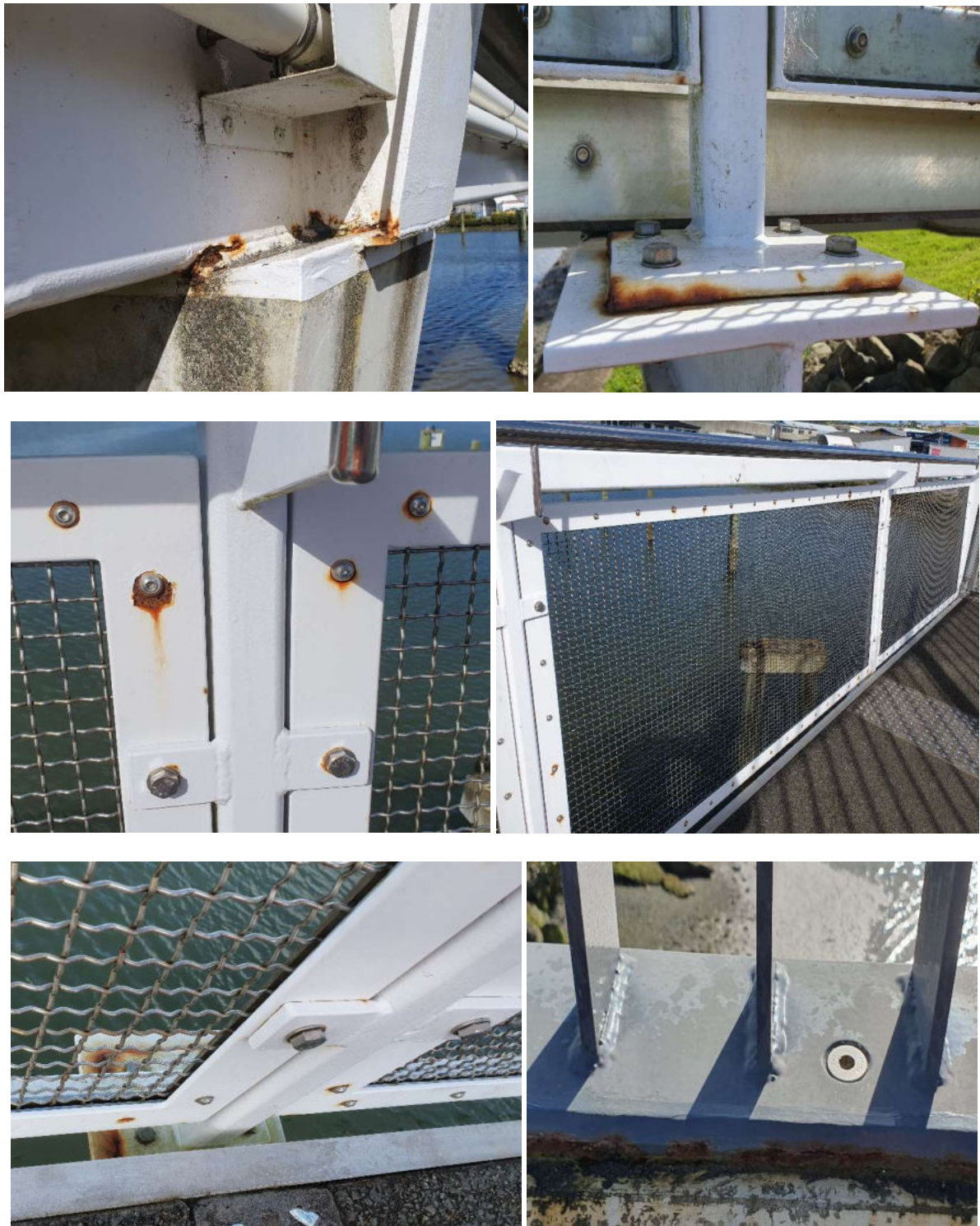
Figure 2-12: Level of deterioration on TMaP and KTTW handrail mounts
