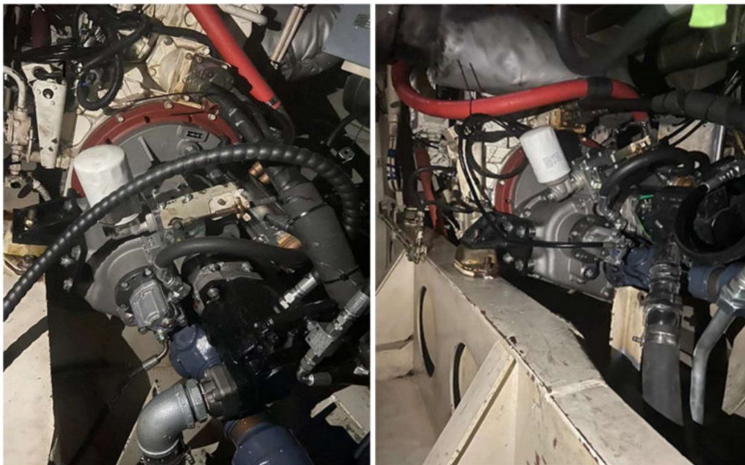
Figure 1-2: Newly installed gearboxes units
