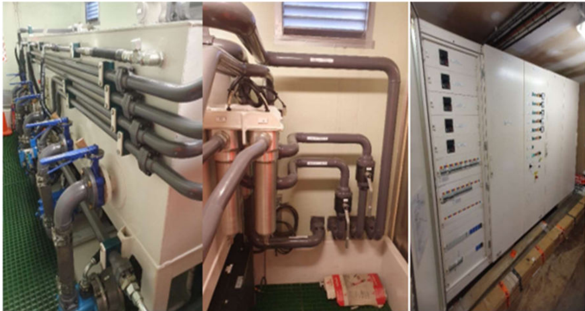
Figure 1-3: Hydraulic & Electrical plant room
