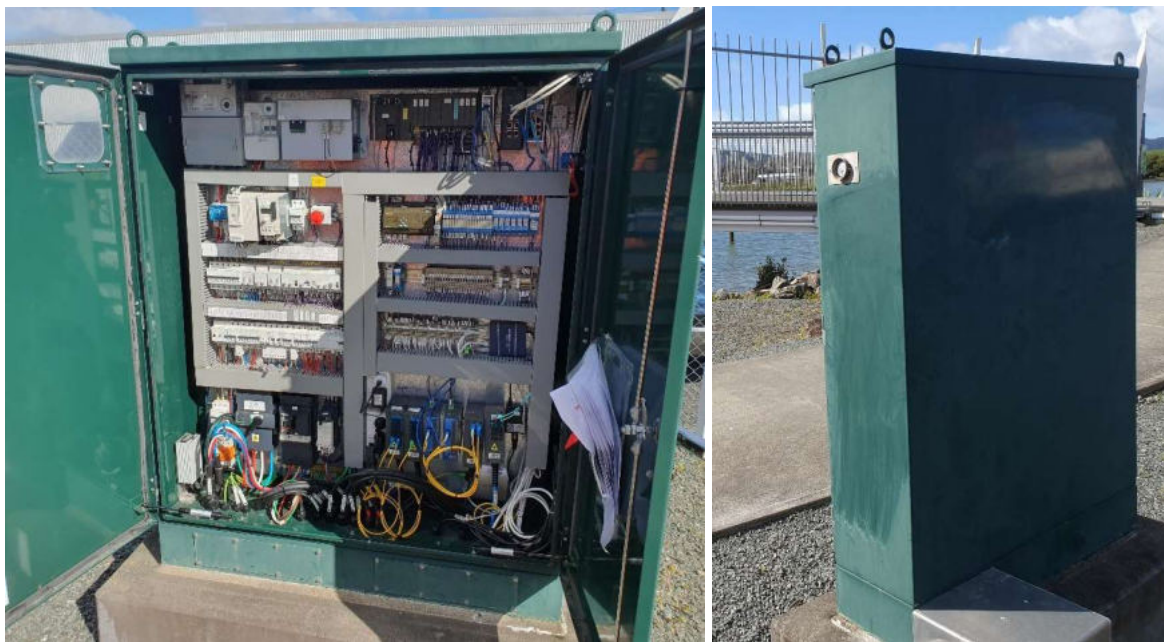
Figure 2-6: Electrical switchboard internal space limitations
