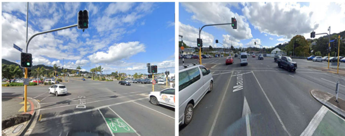
Figure 1-2: Traffic Signal mast arms & lanterns
