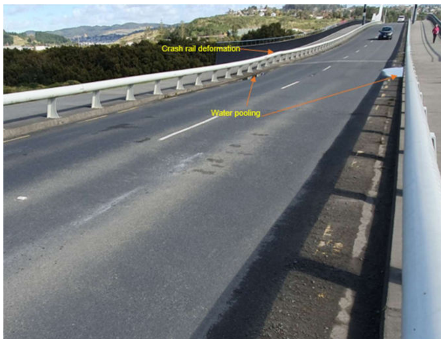
Figure 2-11: Water pooling and the pavement settlement
