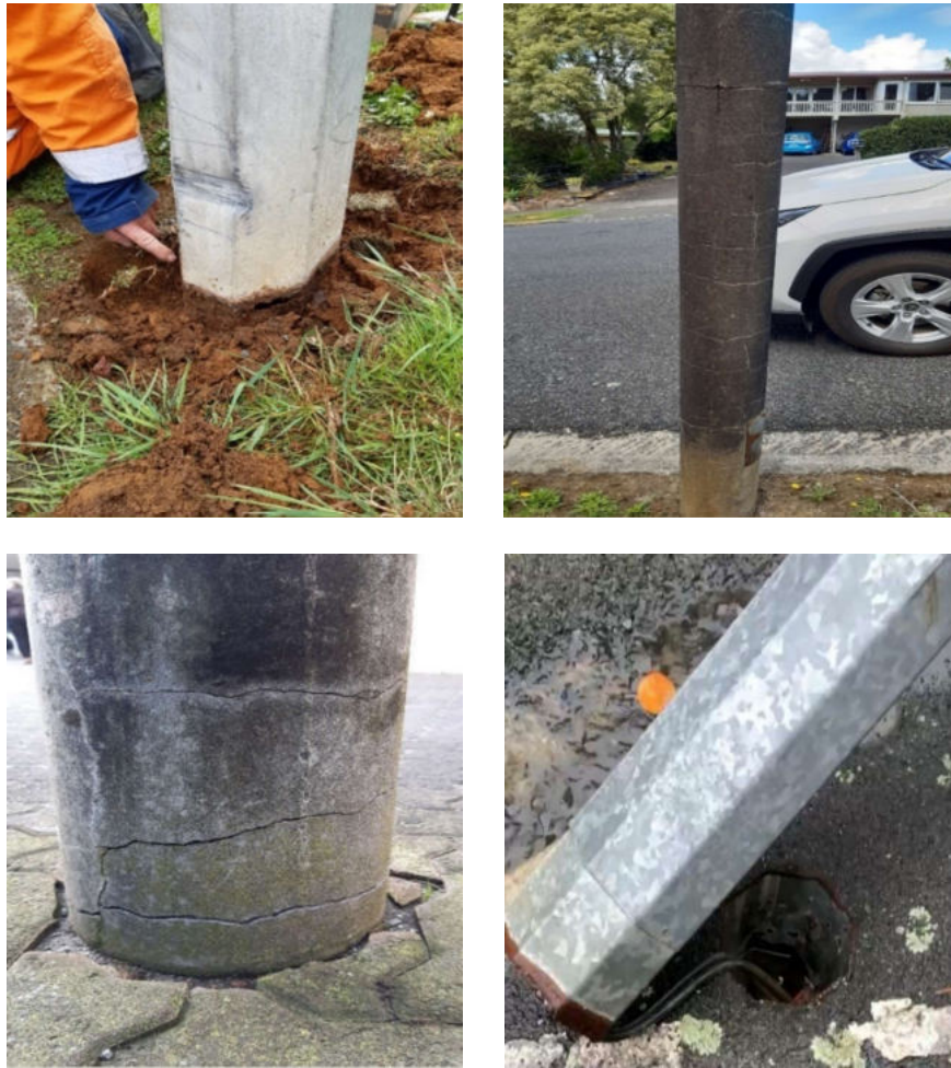
Figure 1-6: failures of steel and concrete streetlight columns
