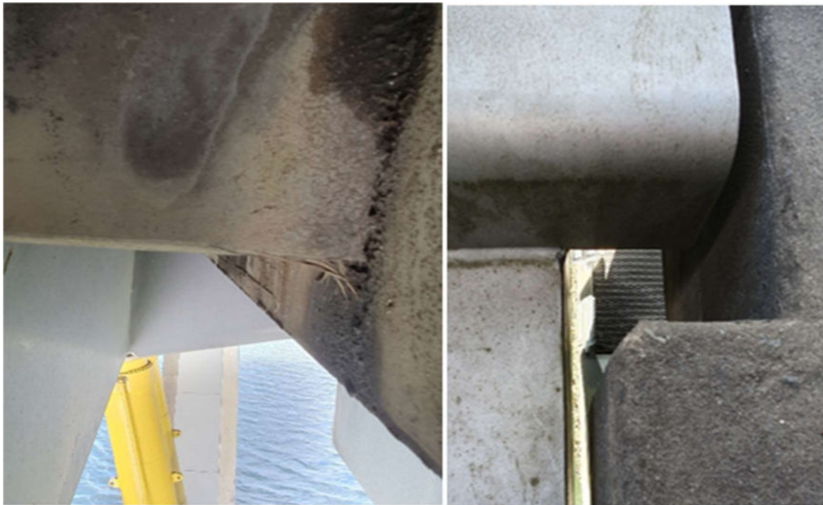
Figure 2-13: Gap between the bridge lifting section and fixed portion and water tracking marks on the piers
