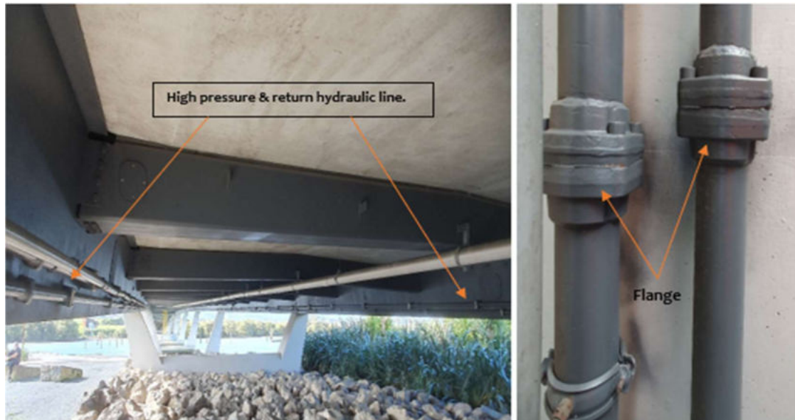
Figure 2-4: Hydraulic pipe network under the bridge
