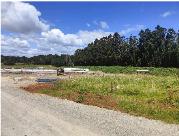
Figure 11: Slab for boat building factory (is further along in build at present)
