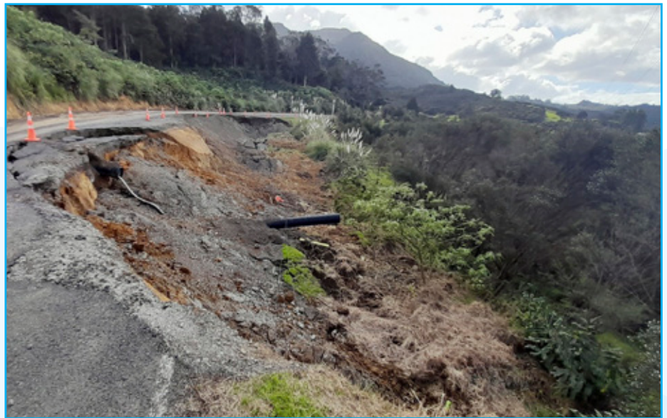
West Coast Road in Panguru was reduced to one lane by a major underslip in August 2022.
