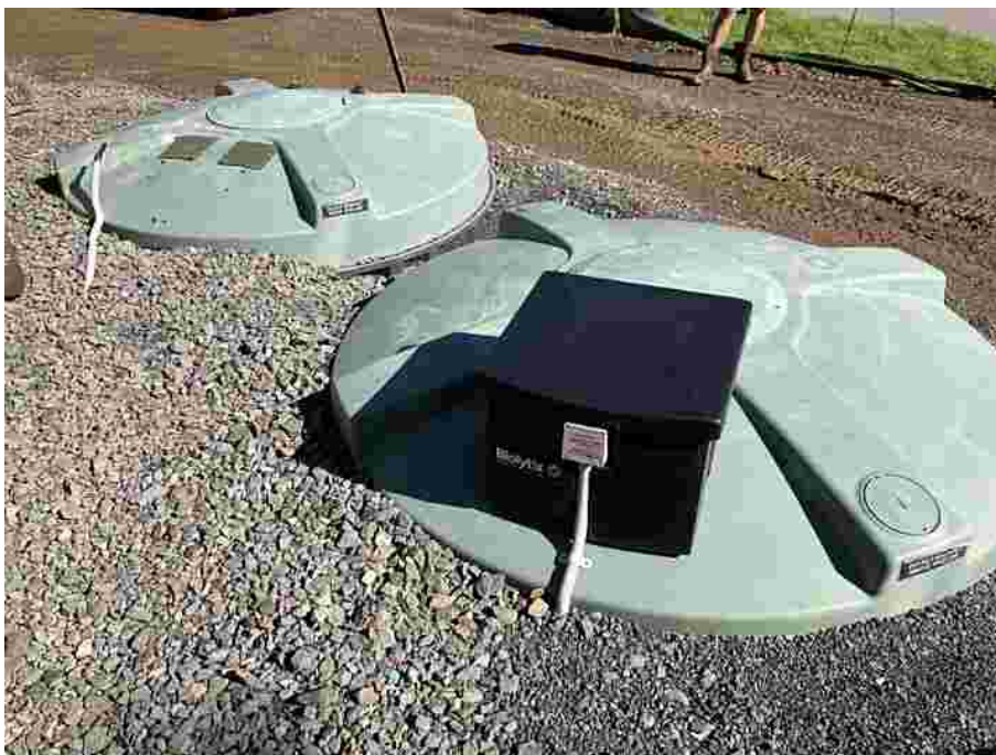
Figure 19: Kingfish Lodge Biolytix Wastewater Treatment unit (at southern end)
