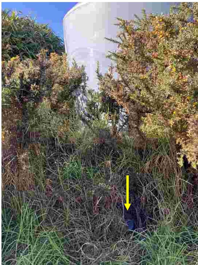
Figure 12: Lot 1 Rainwater tank overflow outlet pipe on western side
