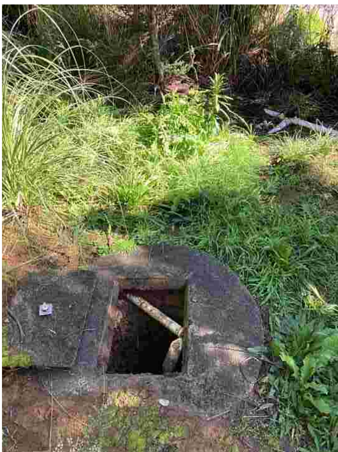
Figure 21: Kingfish Lodge Typical Wastewater disposal soakage pit at higher elevation RL=52m
