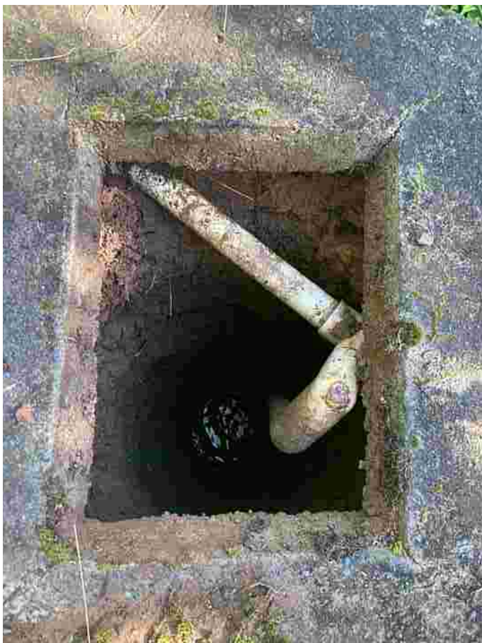
Figure 22: Kingfish Lodge Typical Wastewater disposal soakage pit
