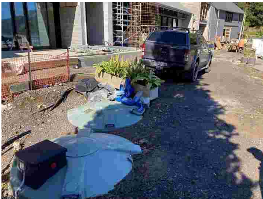
Figure 20: Kingfish Lodge Biolytix Wastewater Treatment unit (at northern end)
