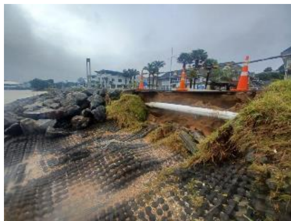
Marsden Rd Paihia footpath damage
