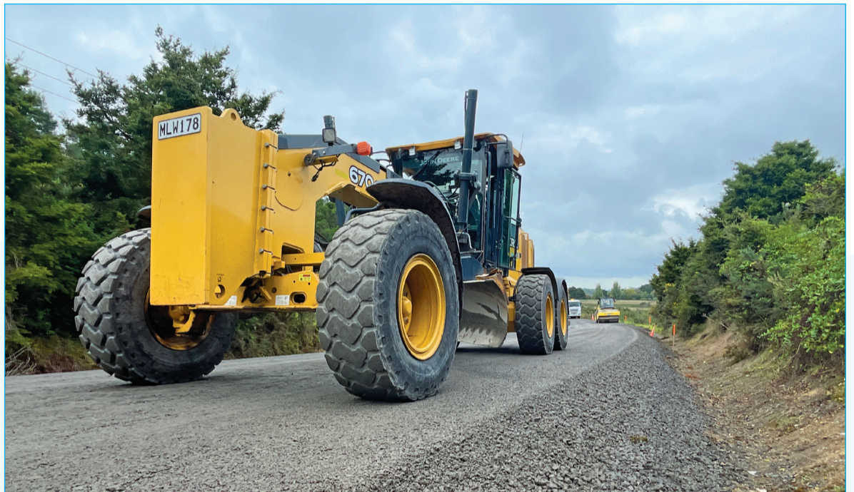
Fulton Hogan has been awarded the contract for the northern section of the network, and Ventia has the southern area contract.
