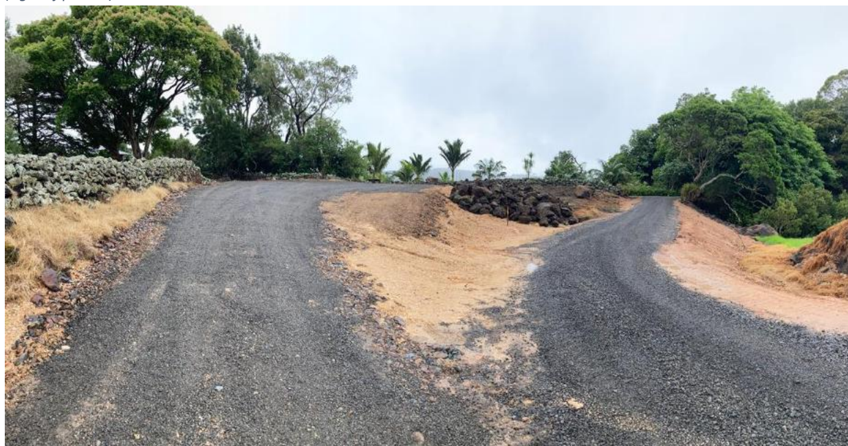
Figure 3: Photograph showing recent earthworks within Lot 2 (left of picture) and raised accessway to join Crown Grant Road (right of picture)
