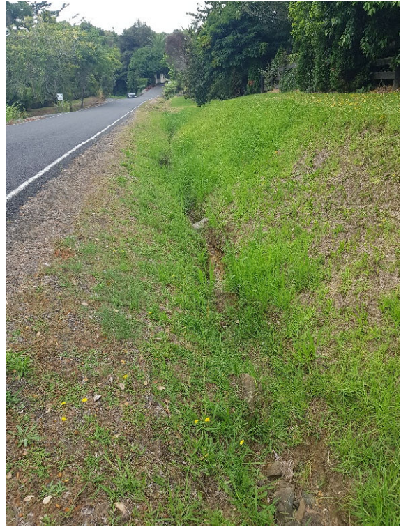
Roadside drain outside 80A Pa Rd – Looking North-east
