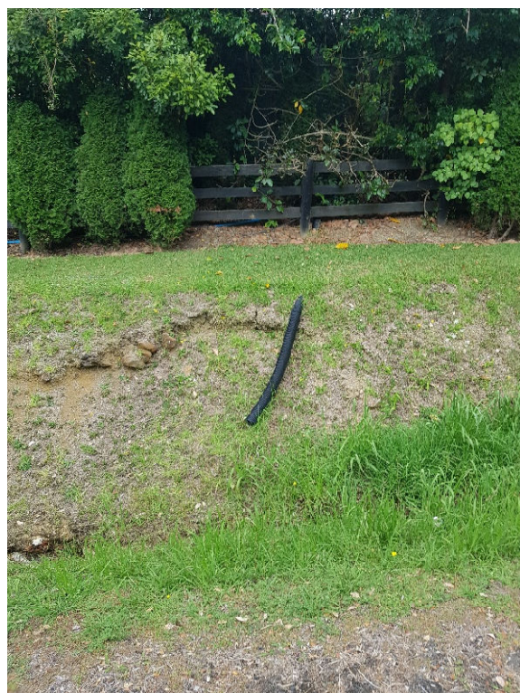
Existing overflow outlet from water tanks
