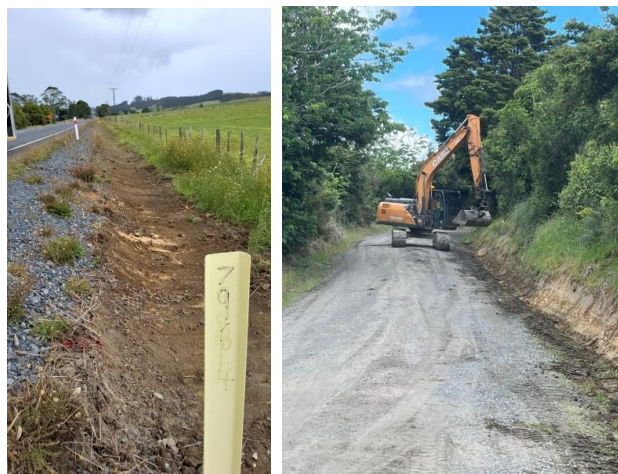
Te Ahu Ahu Road / Taheke Road – Water Tabling
