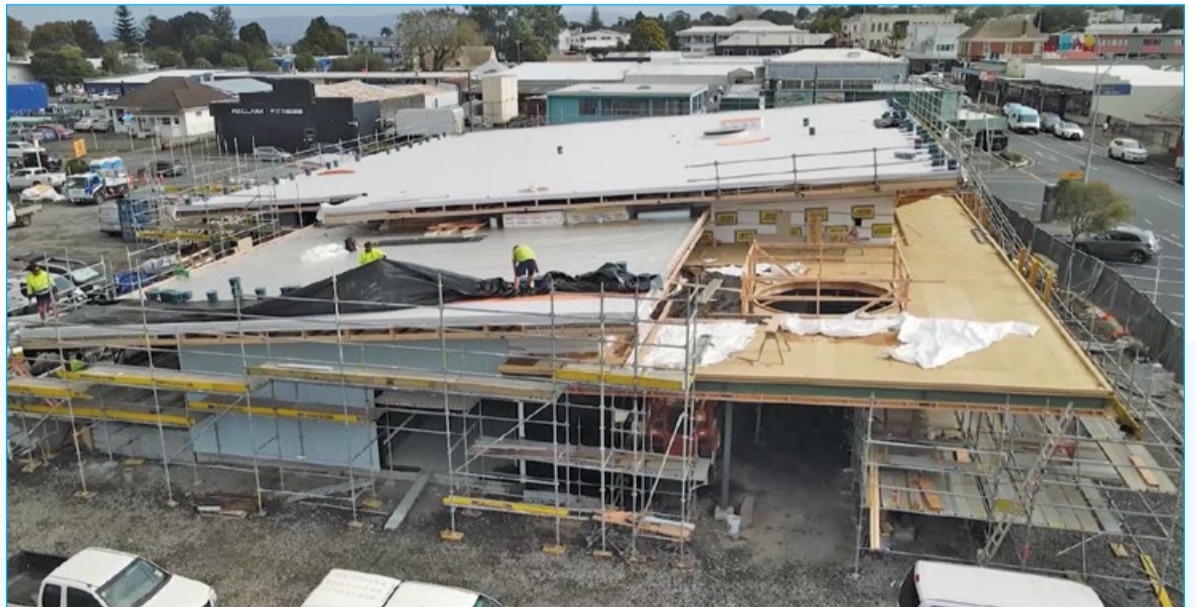
Adding the roof and external wall cladding mark a significant milestone in the construction of Kaikohe's new library and civic hub.
