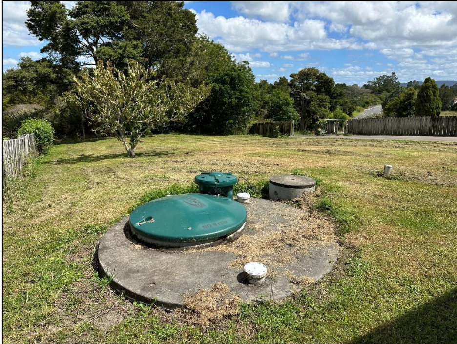
Figure 11. Advance Secondary Treatment Plant
