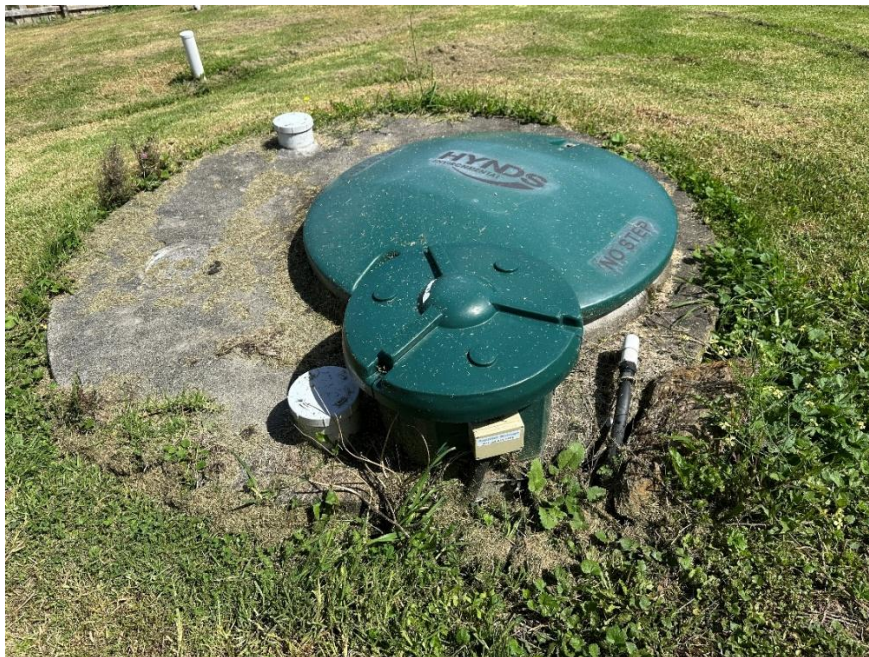
Figure 5. Advanced Secondary Treatment Plant
