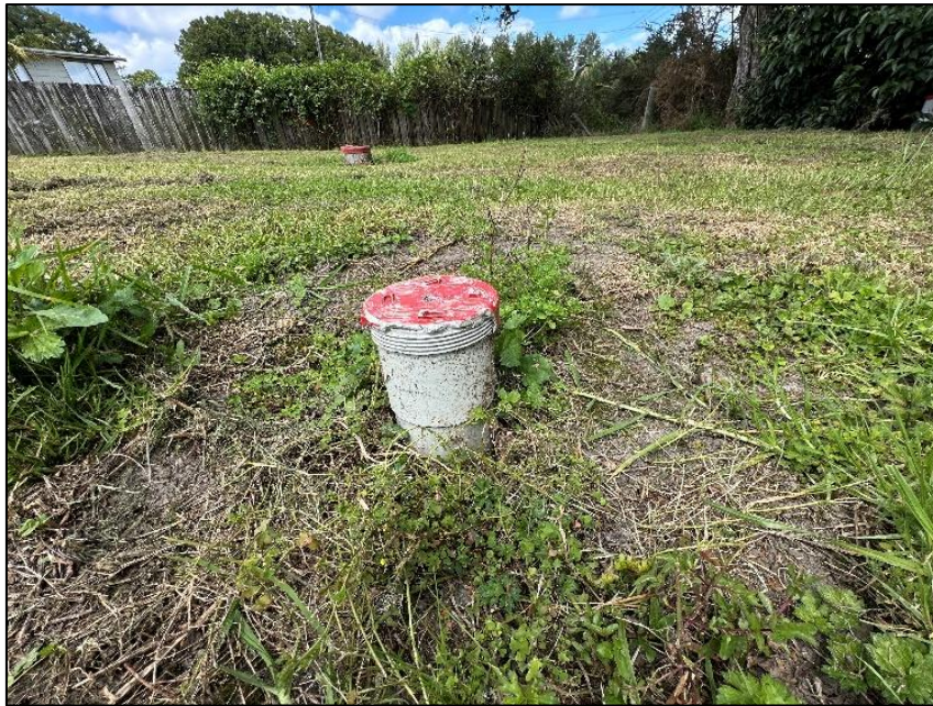
Figure 13. Damaged Subsoil Drain Vent Cap
