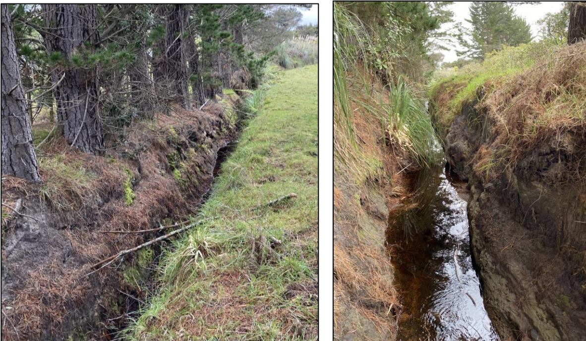
Figure 6 – Deep drain inside property on boundary with Sweetwater Road
