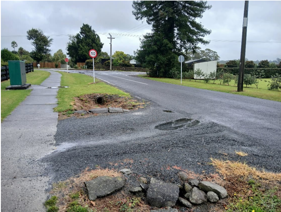
Figure 8: View along Kendall Road toward Landing Road from the site entrance, showing the existing swale/culverts.
