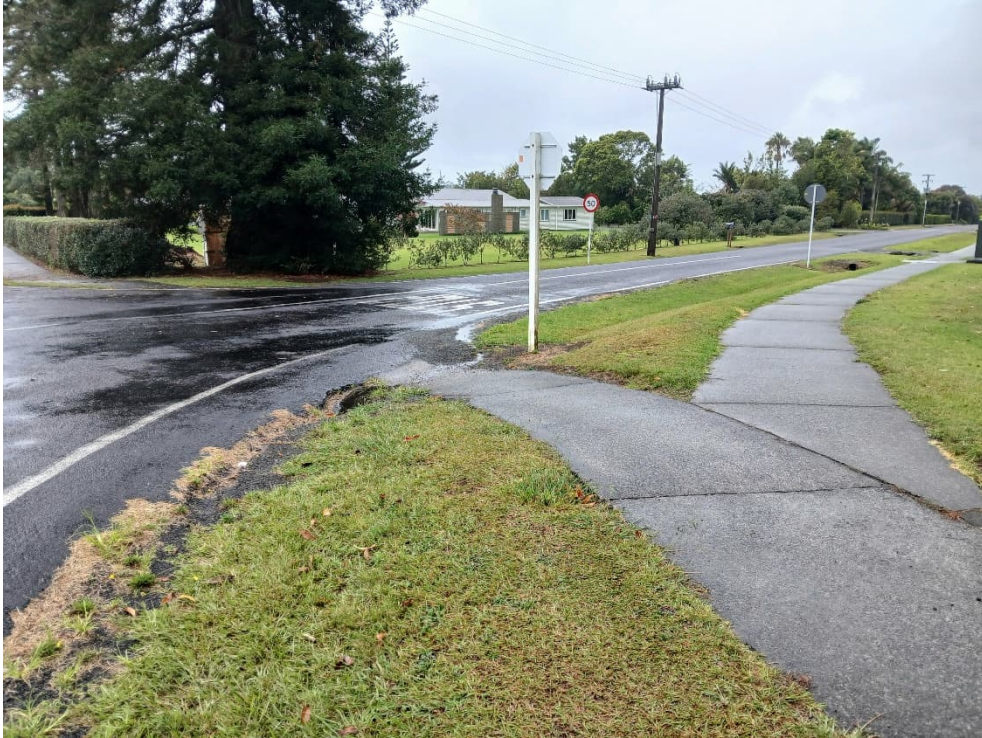
Figure 10: View to the north of the intersection of Kendall and Landing Roads, showing the existing swale and drainage.
