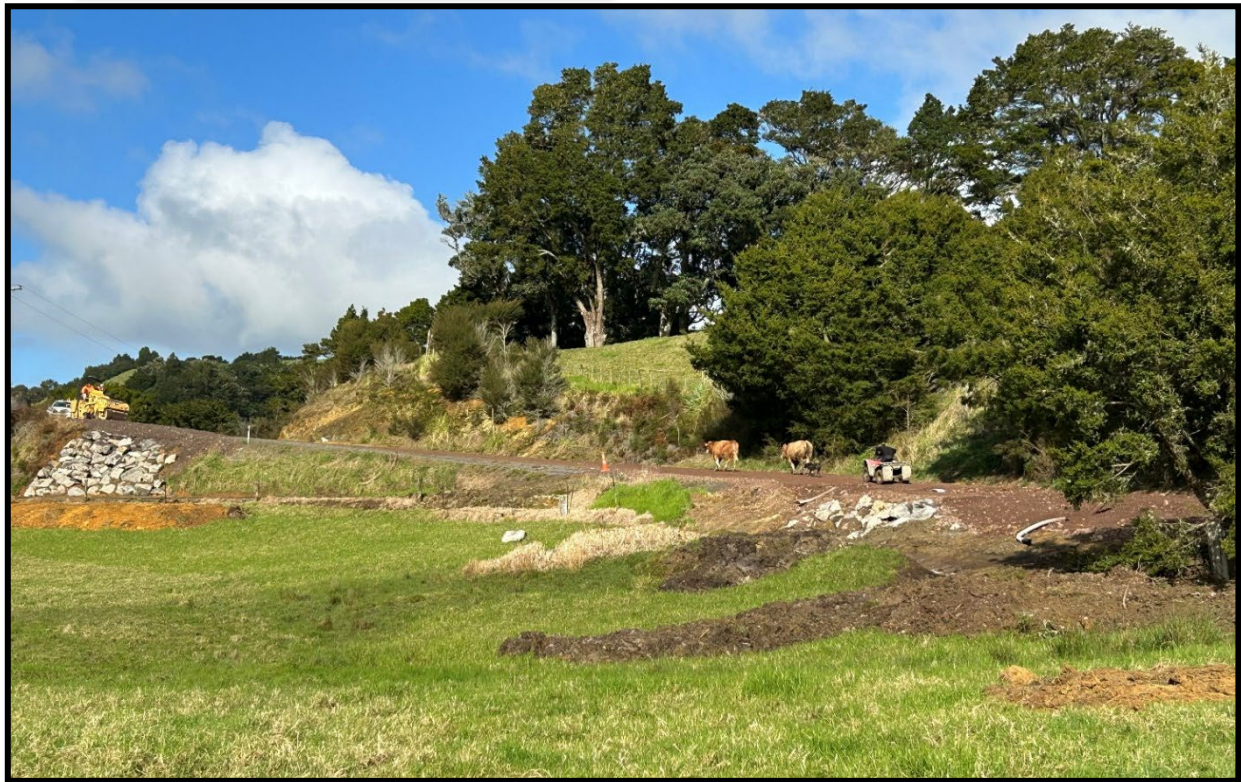
Marlow Rd Under slip (local traffic moving through site) note to the left a second small drop out type slip having been rock armoured.
