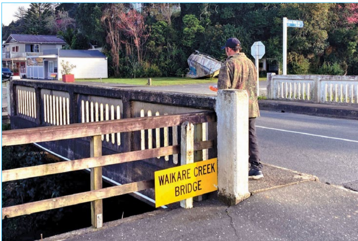
Preliminary work is getting under way on a new footbridge at Kāeo to improve safety for pedestrians in the Far North town.
