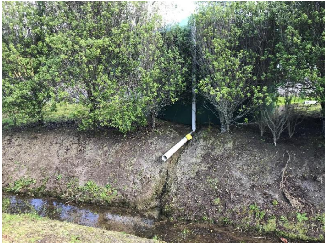
Figure 19 - Existing overflow from water tank into drainage easement
