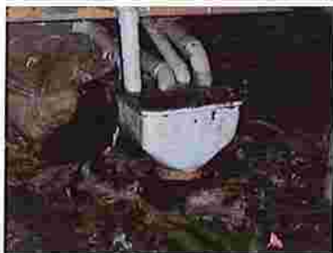
Backup to gully trap from clogged tank
