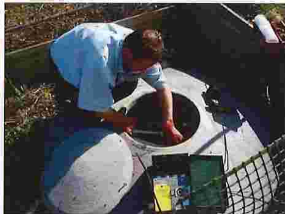
Servicing an advanced wastewater treatment unit
