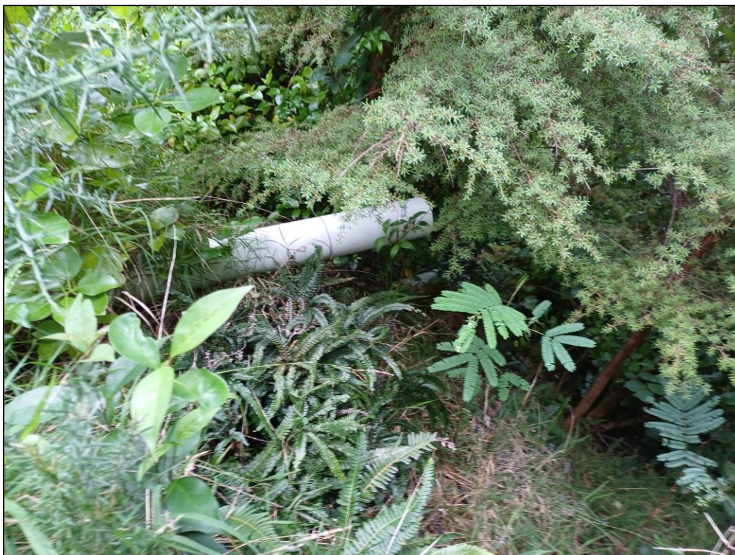
Figure 4 - Outlet from eastern tanks
