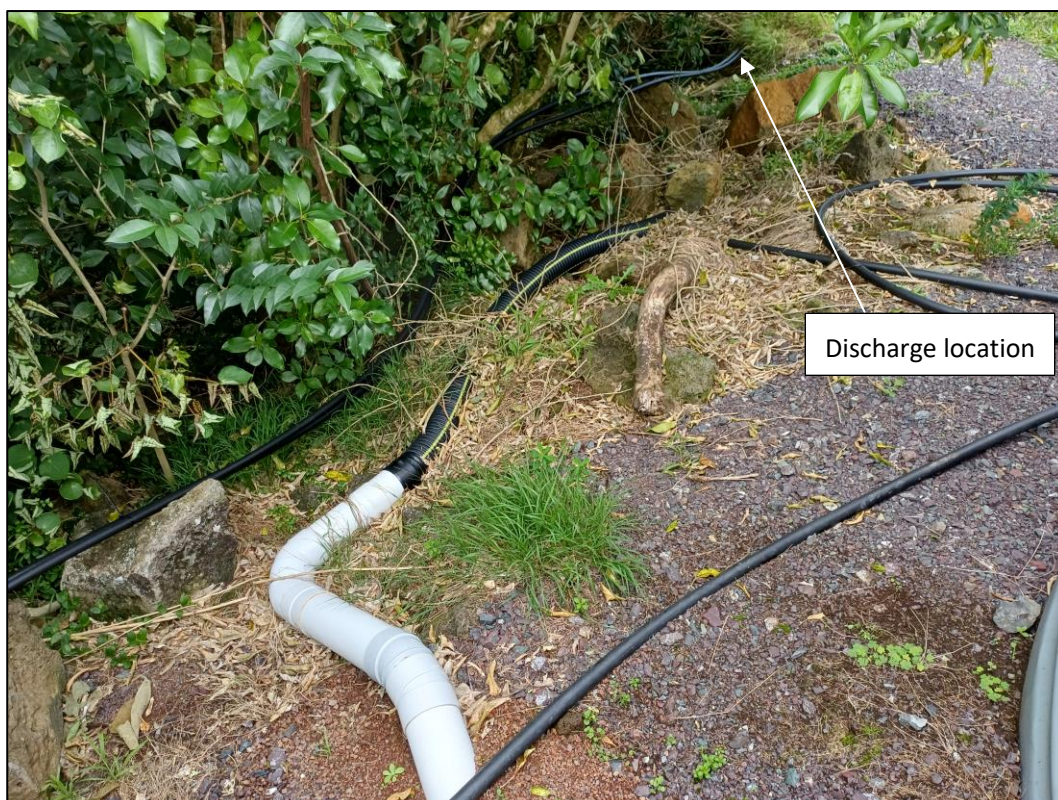
Figure 5 - Outlet from western tanks
