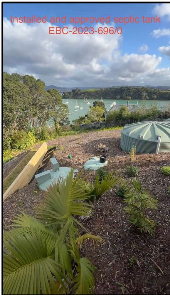
Figure 6: Approved onsite wastewater system under RC 2230465 - RMALUC.
