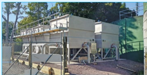
State-of-the-art clarifiers now treat Kerikeri-Waipapa water supplies.
