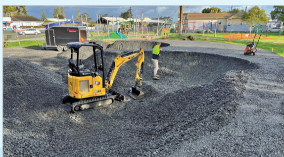
The pump track will be in addition to other Awanui park upgrades.
