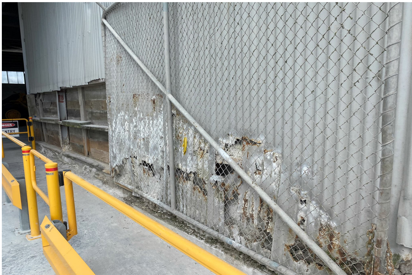
Figure 6. Deteriorated corrugated iron cladding.
