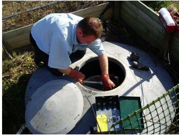
Servicing an advanced wastewater treatment unit
