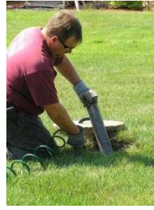
Lifting and hosing down effluent outlet filter
