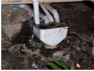
Backup to gully trap from clogged tank
