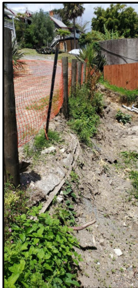
Figure 9: Existing slippage into 21 Baker Street.
