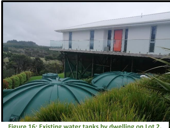
Figure 16: Existing water tanks by dwelling on Lot 2.
