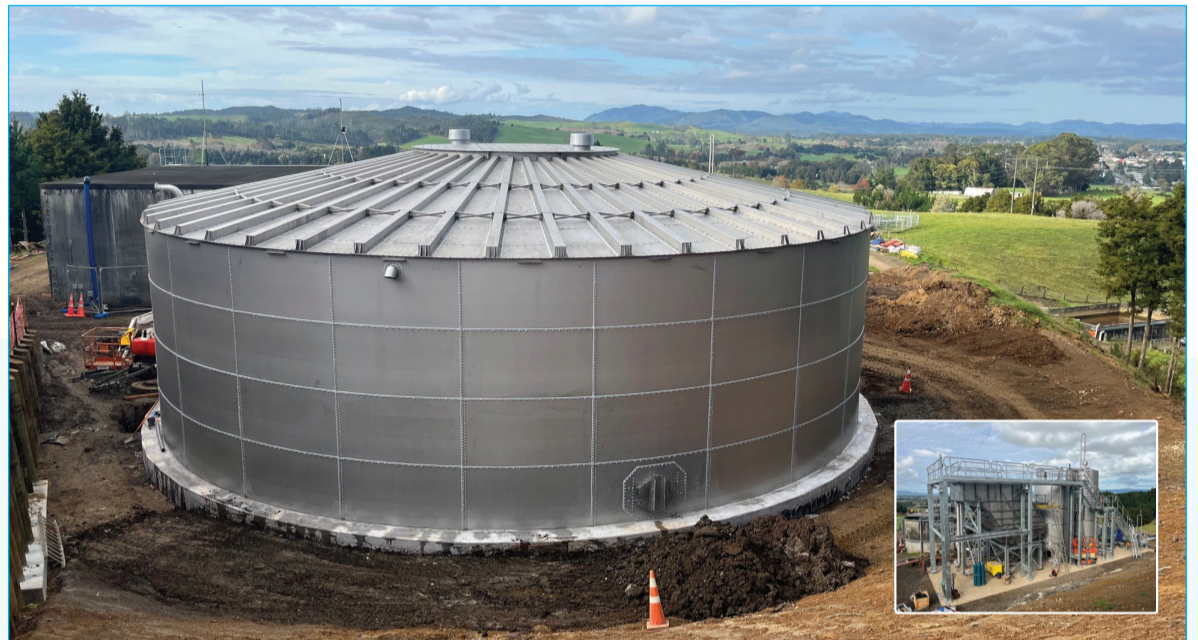
The new 1.5 million-litre storage reservoir has a lifespan of 100 years and supplies Kaikohe and Ngāwhā.
