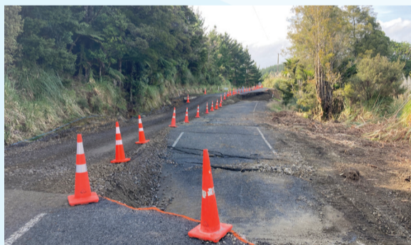
A single lane has reopened at the site of a West Coast Rd slip.
