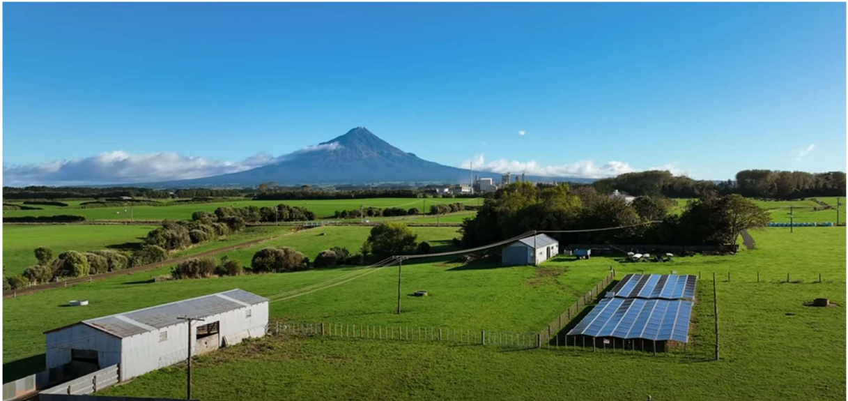
Figure 3. Example of a similar sized solar install in Kapuni, South Taranaki
