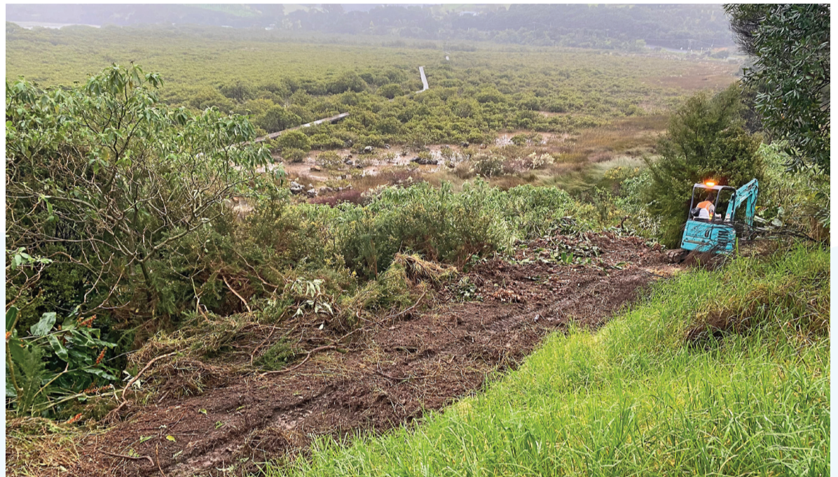
Cycleway construction is community-led and breaking new ground between Russell and Ōkiato.
