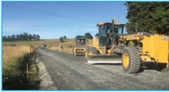
Sealing sections of road near homes and public facilities reduces the harmful impacts dust has on people's health.
