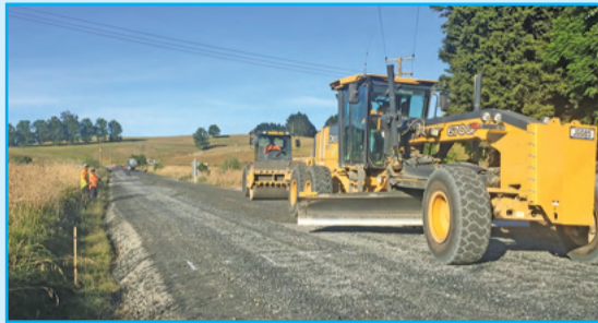
Most sealing work on Council roads is undertaken during warmer weather between November and May.
